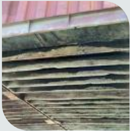
Crossbeams collect soil and provide refuge for pests.
