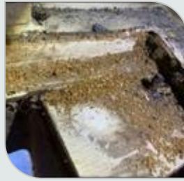
Contamination can go undetected under floorboards.
