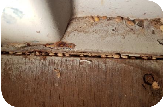
Gaps between floorboard and container wall
