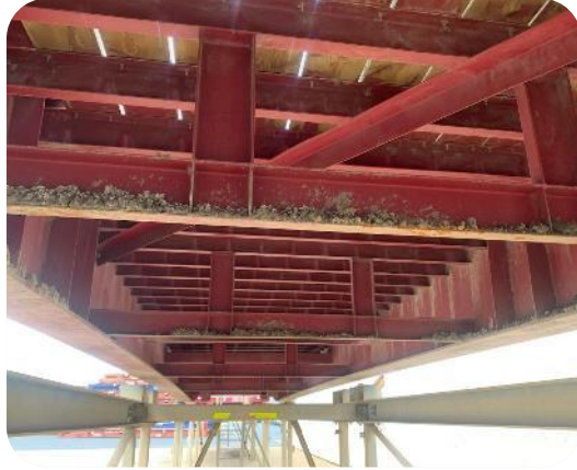
Soil on rails under the container
