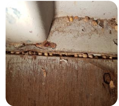
Seed caught in interface between wall and floor
