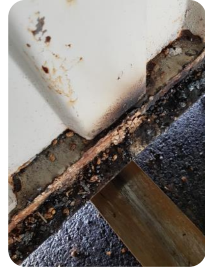
Seeds and debris on interface between floor and wall
