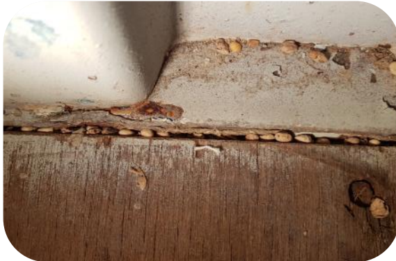
Gaps between floorboard and container wall
