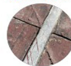
cracks and crevices
