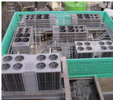
Air conditioning facility
