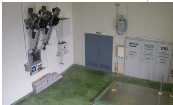
(4) Exterior of the irradiation room: manipulator and lead glass (in the middle), water treatment control panel and sub-pool for temporary storage of Cobalt 60 source during maintenance (on the right).
