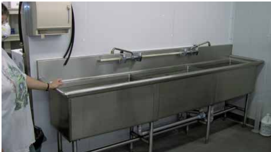
FIGURE 26 Stainless-steel tanks (3) for immersion of egg sheets in a disinfecting solution and then rinsing in water (OKSIR facility, Osoyoos, Canada)
